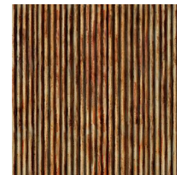
EXTERIOR CLADDING CORRUGATED METAL - DISTRESSED
