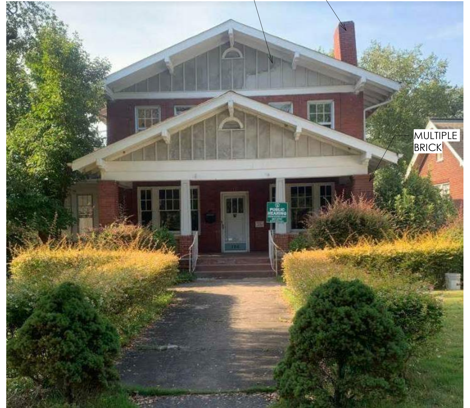
PLASTERED GABLES IN NEED OF REPAIR
