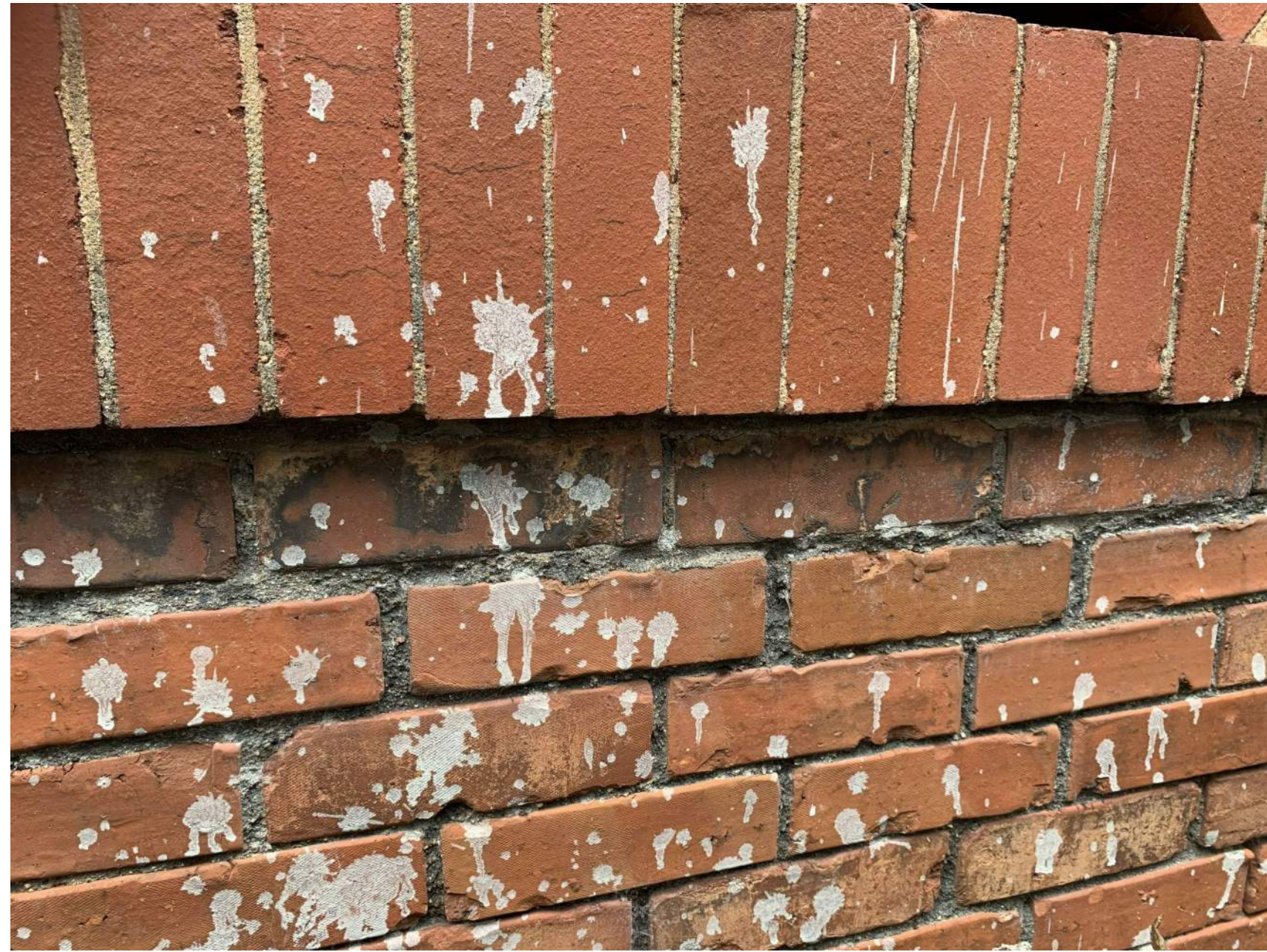
REPOINTING OF BRICK NEEDED & PAINT STAINS
