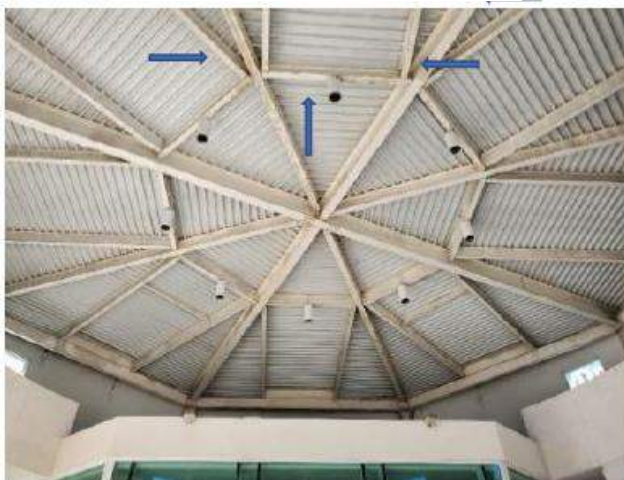
Ceiling Lighting (8 total)
