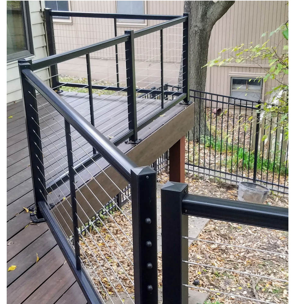
EXTERIOR CABLE RAILING
