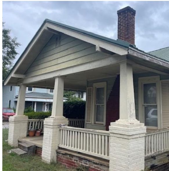
Side Porch Conditions
