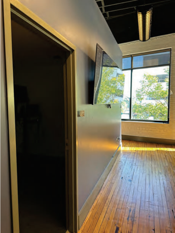
Photo 11: Original 2nd story wood floors with oil stains
