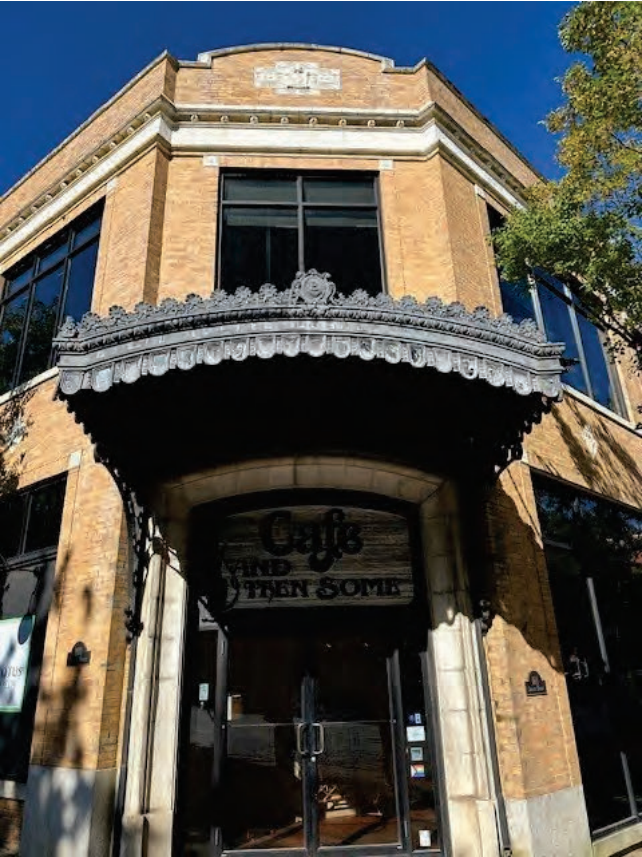
Photo 2: Original metal awning front view
